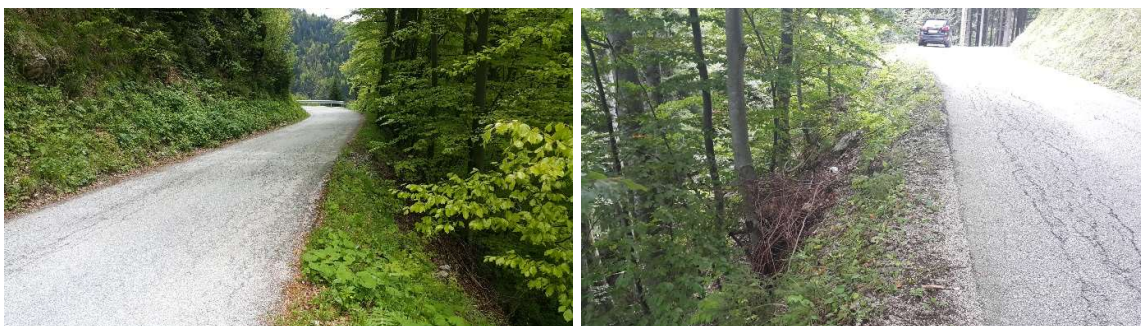
FOTO 13 in 14: Usad v nasipu nad evidentnim plazom v km 2.680
